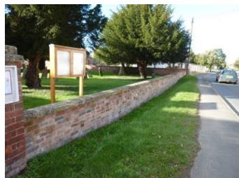
Above: the before and after pictures of the wall at St David's, Newbold on Stour
